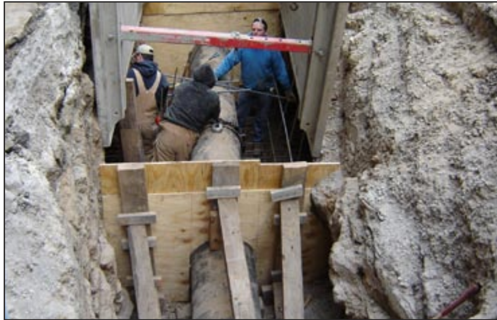
Approximately 1,000 linear feet of existing 20" cast iron pipe water main was relocated and replaced with 20" ductile iron pipe on 14th Street between Central Avenue and Baltimore Avenue to make way for construction of an underground walkway access to Bartle Hall. This is part of the Bartle Hall Ballroom Expansion Project. The line relocation cost was $200,000.
